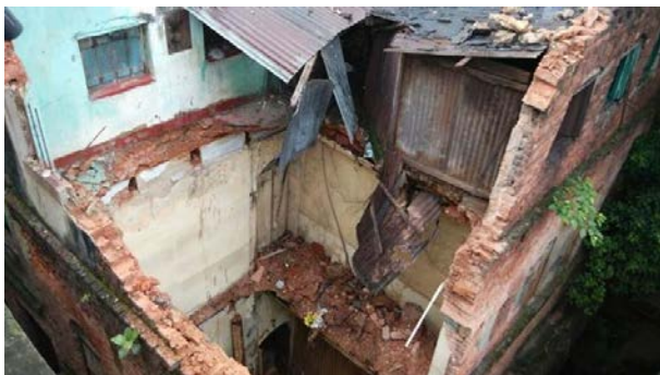
Photo: Incident of Dilapidate Building Collapse at Burrabazar (Source: NDTV)
